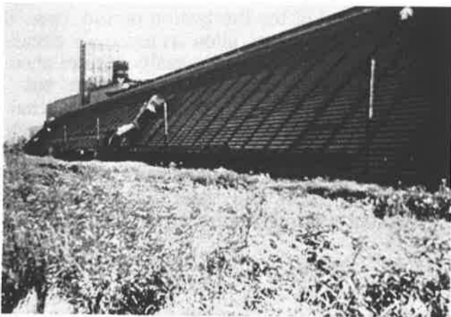
Figure 18. Recirculating ducts on storage building
