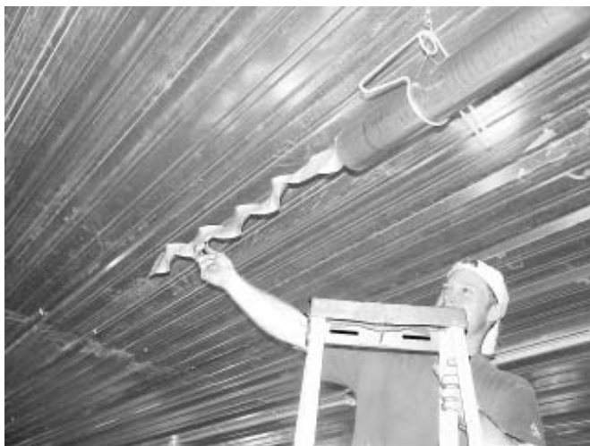
Workman installing element designed to even out temperature from combustion chamber to end of tubing. The device, installed in the last 10-15 feet of tubing, acts as a heat sink to extract heat from the exhaust gases and convert it into radiant energy. Radiant tube manufacturers use various devices of this kind to help improve the radiating efficiency of the heater. Note bracket on tubing that will be used for installing the reflector/heat shield to protect house ceiling and direct radiant energy toward the birds and the litter.
