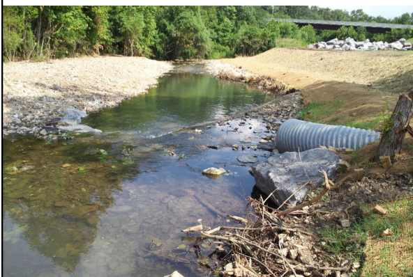
Log J-Hook Vane: Downstream of stormwater pipe
