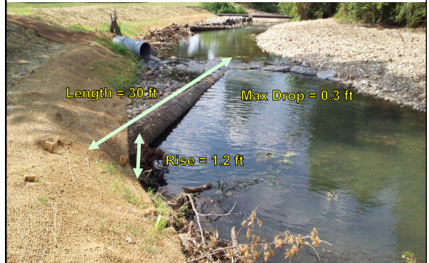
Log J-Hook Vane: Flow direction, bank protection, habitat Arm slope = 1.2 / 30 = 4\% ; Arm angle = 25 degrees
