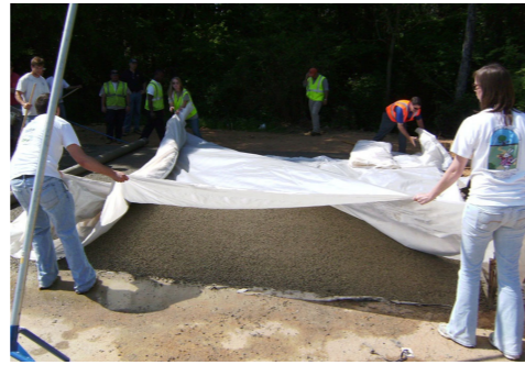
Figure 6.13. Placing plastic sheeting over pervious concrete at Duck Samford Park, Auburn, AL. (Photo courtesy of Michael Hein.)
