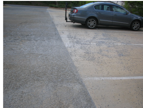
Figure 6.14. Surface raveling, Auburn, AL.
