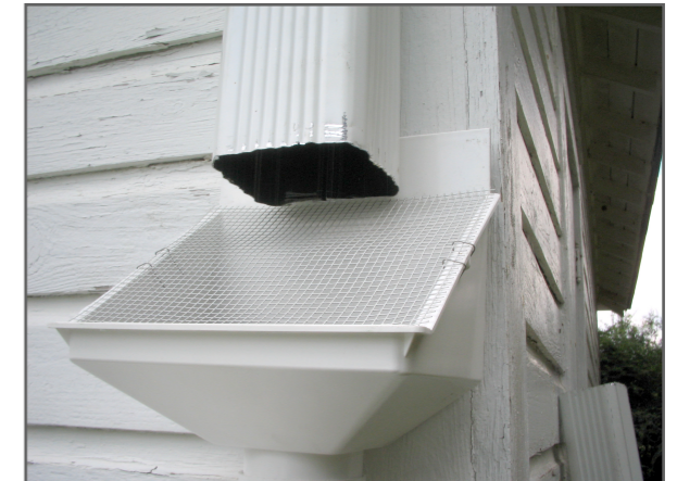
Figure 9.5. Rain head clean of debris.
