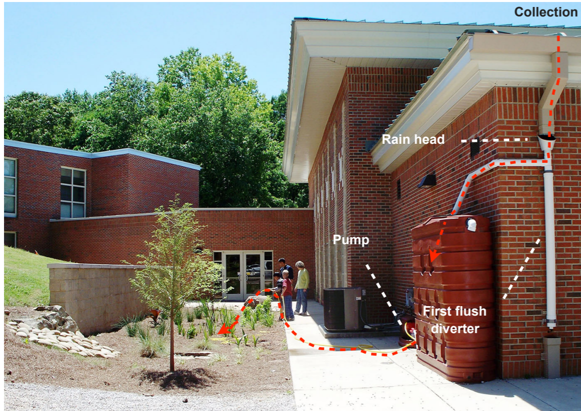
Figure 9.6. The rainwater collection system can be a discrete part of buildings and landscapes. Cary Woods Elementary School, Auburn, AL.
