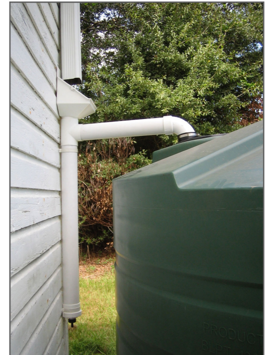
Figure 9.3. Rain head and first flush diverter system, Summerdale, AL.
