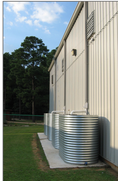
Figure 9.2. Rainwater harvesting system at Boykin Community Center, Auburn, AL.
