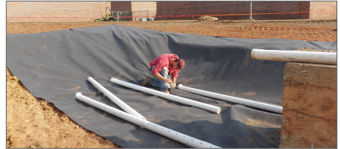
Figure 4.4. Underdrain installation in BRC at East Smiths Station Elementary School, Smiths Station, AL.
