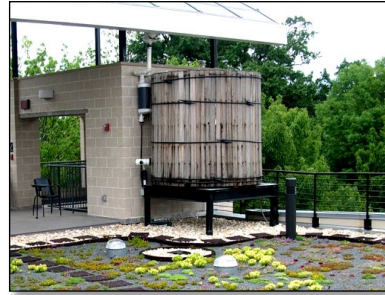
Cistern & Green Roof - Southface
