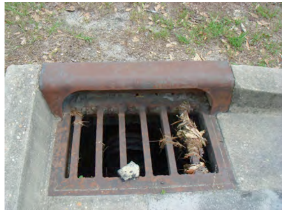
Figure 15. Storm Drain Needs Inlet Protection on CHS Campus.
