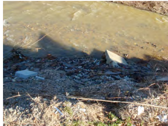
Figure 13. Concrete and Other Materials are Tossed on to Mill Creek Streambanks to Stabilize.
