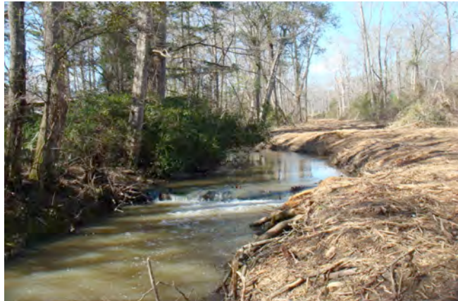
Figure 12. Forested Buffer Lost on Mill Creek During Sewer Trunk Line Installation.
