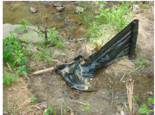
Figure 7. Incorrectly Installed Silt Fence Near Mill Creek.
