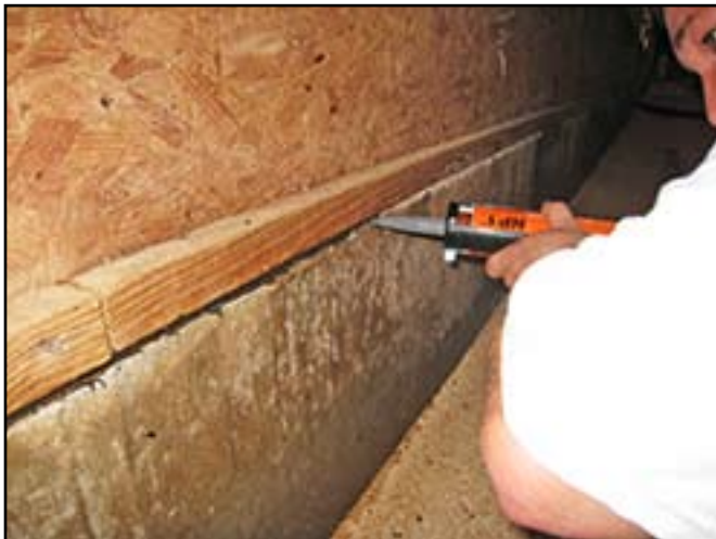
Grower injects foundation sealant using an ordinary caulking gun. Voids must be thoroughly cleaned before applying sealant.
