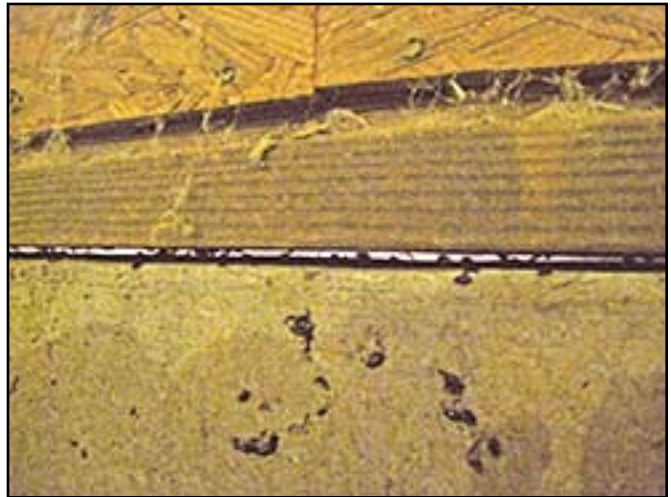
See-through void above foundation of solid wall house may extend around the entire house, an air leak easily equivalent to a wide-open man door.
