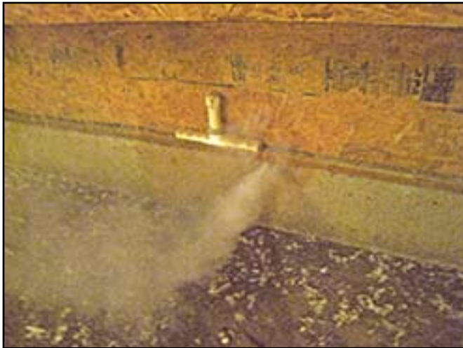
Solid wall house smoke test shows air leak between top of concrete foundation and lumber plate, probably caused by darkling beetle damage.
