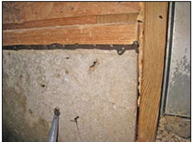
Freshly sealed void should be allowed adequate time to seal per label directions before applying static pressure.
