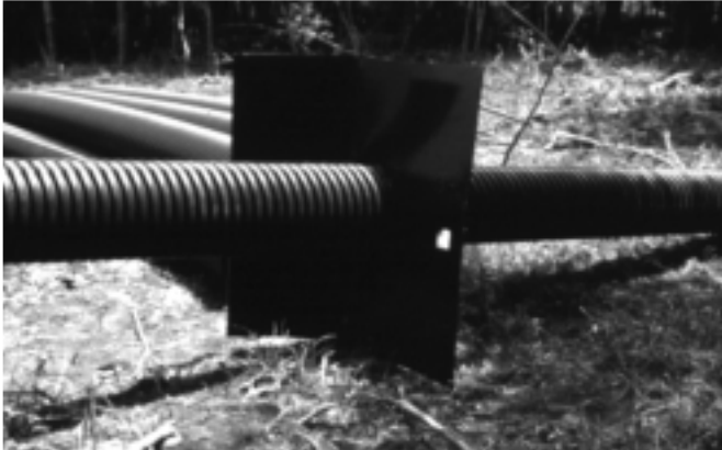
Figure 7. Pipe being prepared for installation through dam (barrel pipe) with antiseep collar attached
